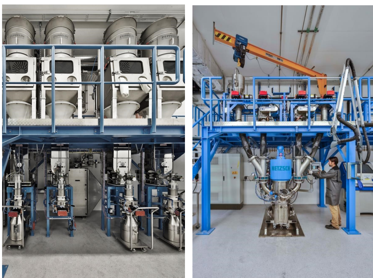
Slurry preparation & mixing station
