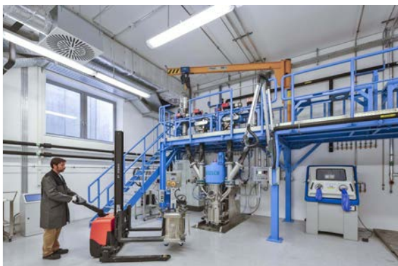
Temperature controlled mixing station for preparing electrode slurries in 60-liter-batches. Source: ZSW/Duckek
